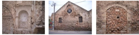
Figure 2: Neoria restoration issues.
