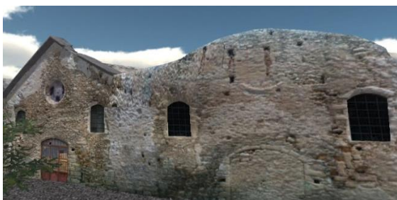
Figure 11: Missing part of the building.
